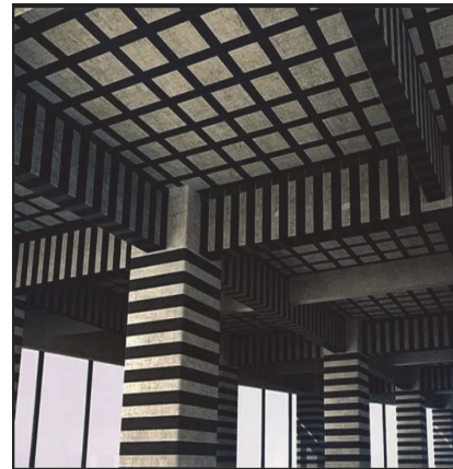
Figure 3. Fiber reinforced polymer jacketing
